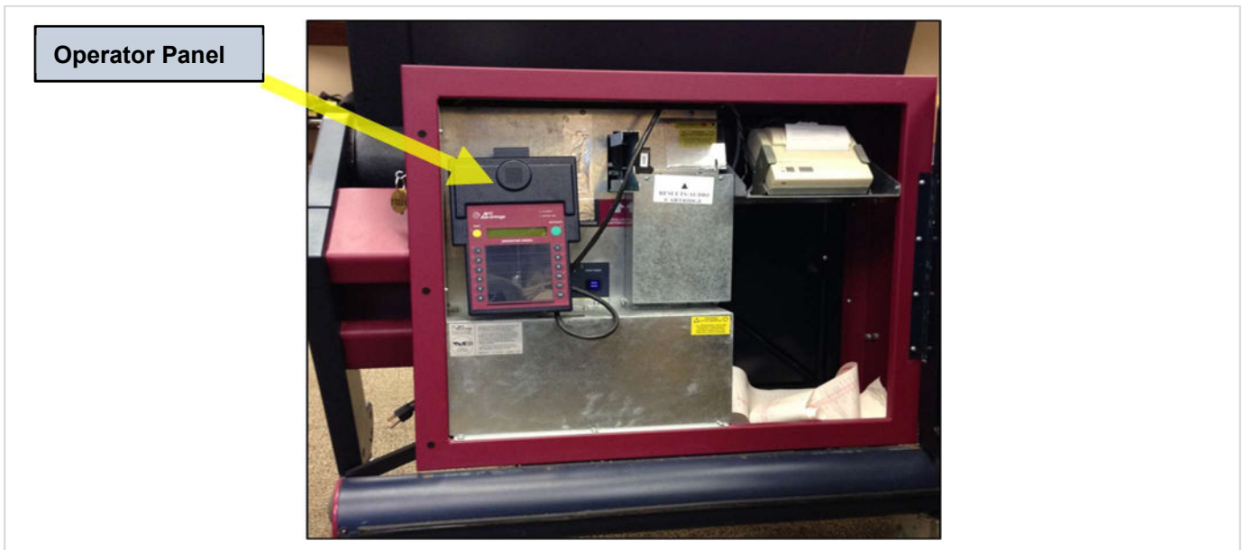
Figure 11: Operator Panel within Back of Unit
